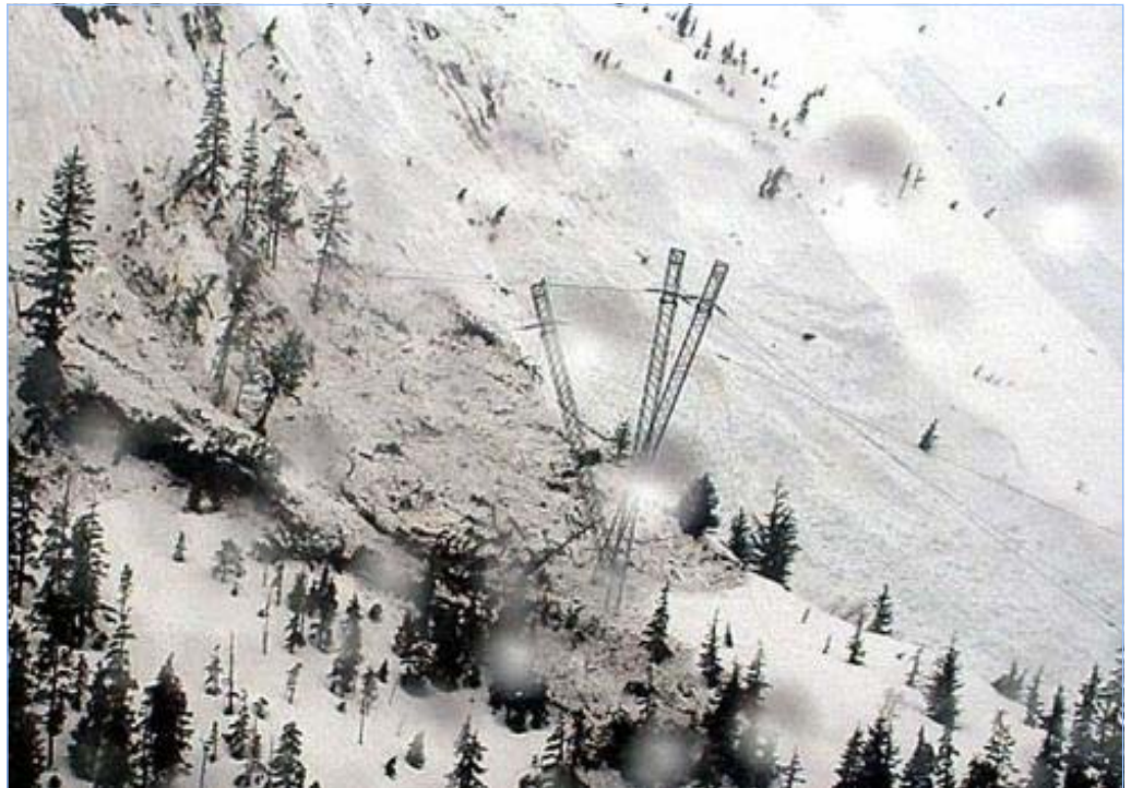
Courtesy Of Mike Laudert / Alaska Electric Light & Power Co. April 16, 2008 - Power disaster: Above, an electric transmission tower that was caught in the avalanche is shown Wednesday about three miles from the Snettisham Power House, about 40 miles south of Juneau. Electric rates in Juneau are expected to rise sharply as Alaska Electric Light & Power Co. switches to diesel power while the structures are repaired.
